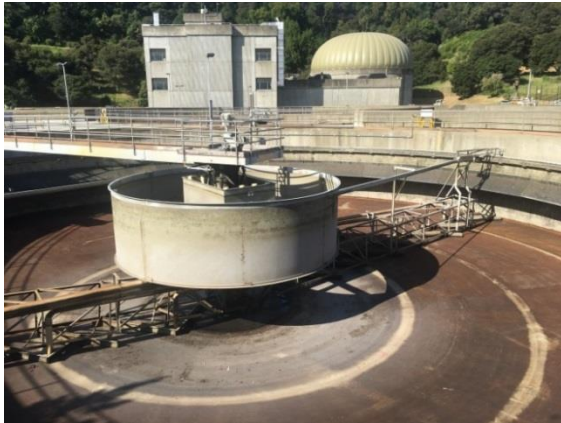
Secondary clarifier internal equipment
