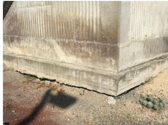
Exposed bottom of process tank
