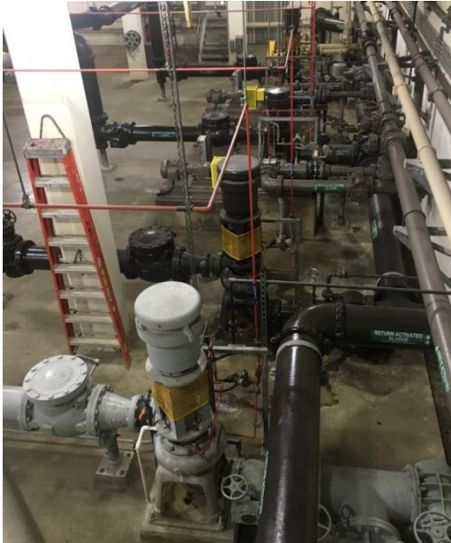
RAS and WAS pumps
