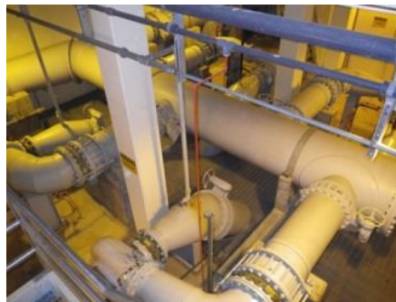
Primary Effluent pipe manifold
