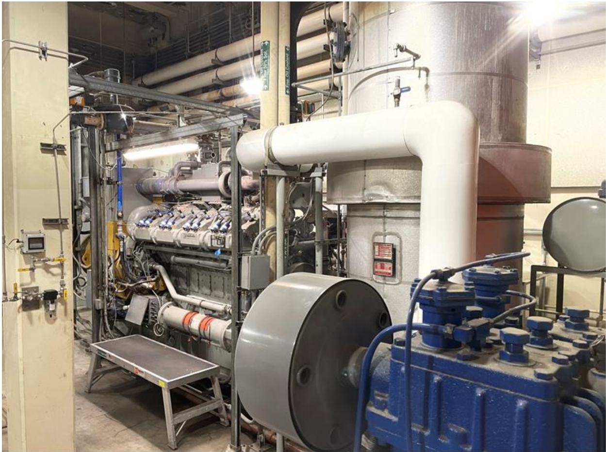
Existing cogeneration system
