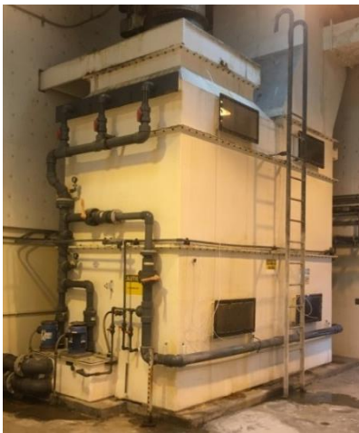
Headworks odor control scrubber
