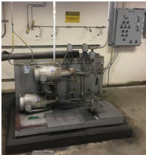
Hydraulic control system
