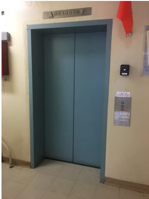
Solids Handling Building Elevator
