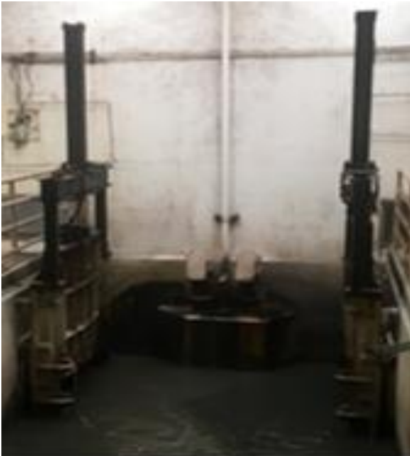
San Rafael and Ross Valley influent gates
