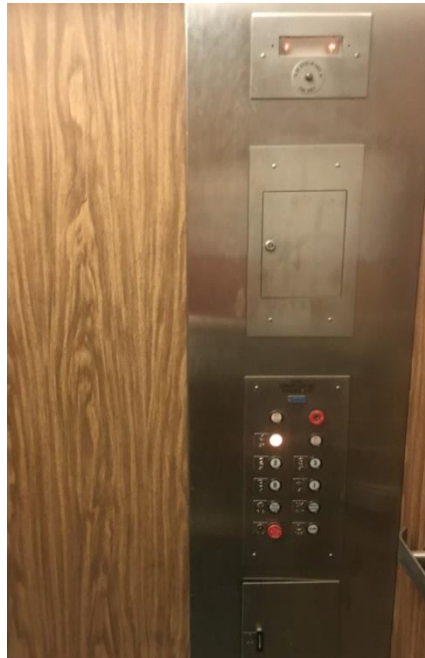
Elevator Control Panel
